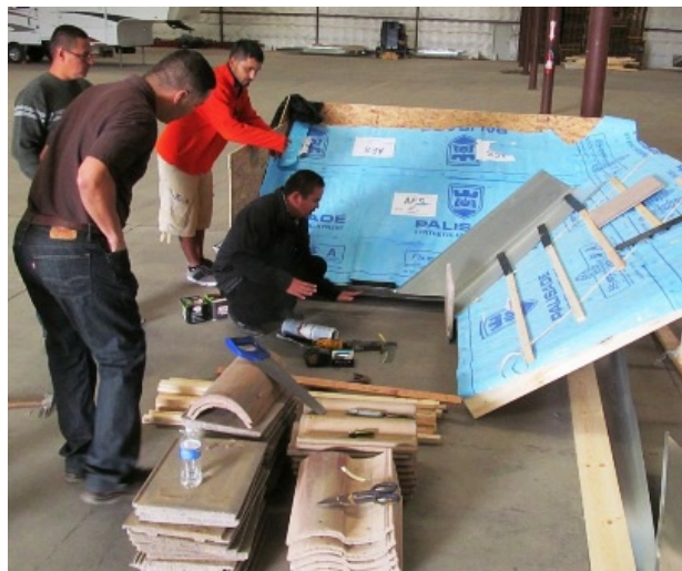
Danny Baca (Chavez Roofing) discusses local techniques with workers from The Roof Depot.
