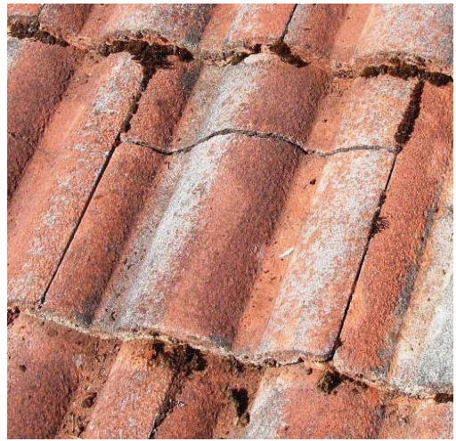
This tile should be replaced.
